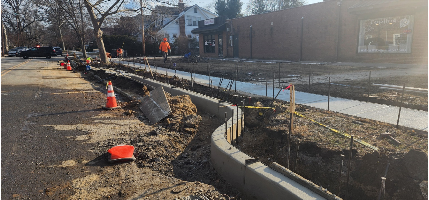
Figure 2: Curbing installed with bump out for additional parking at 9 th and kings highway.
